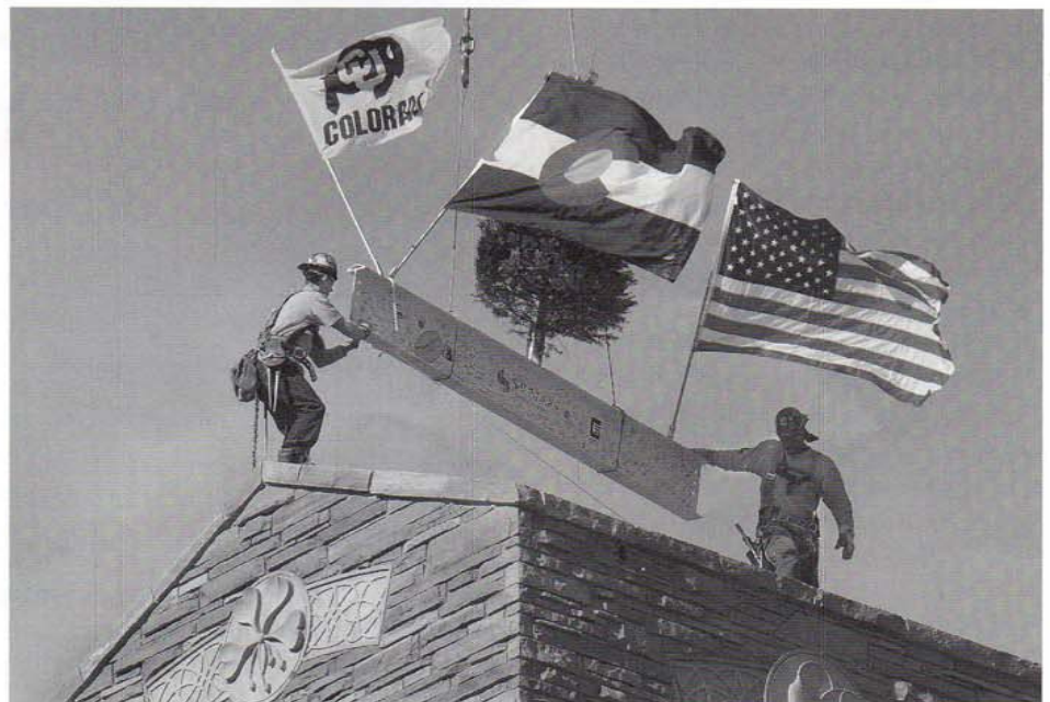
Under windy conditions, two workers with Saunders Construction place the last beam during the “topping-off” ceremony for the 323,000 square foot Center For Community Building.
